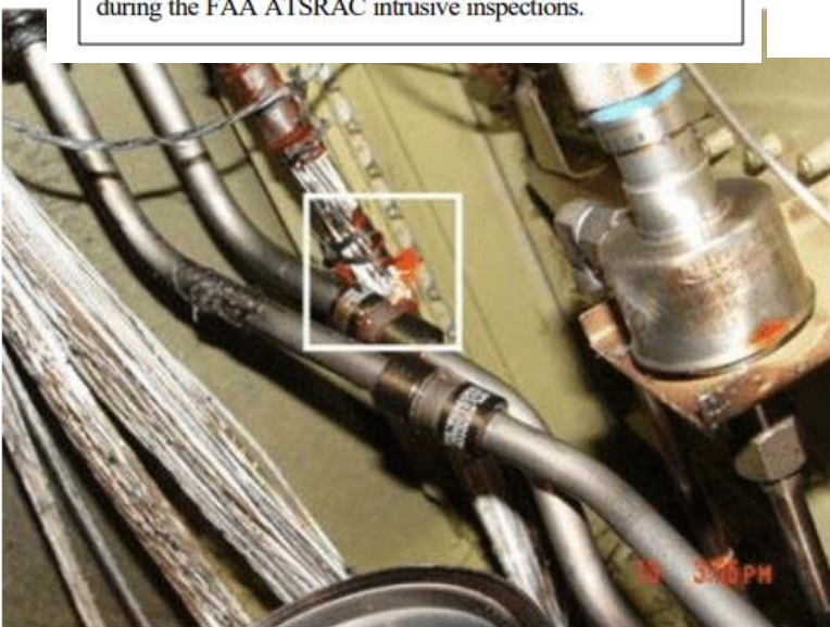
Failure initiation site is shown in the white box. Note that the wire bundle is lying on the hydraulic line. Red anti-chafe tape was used to protect the wiring.
