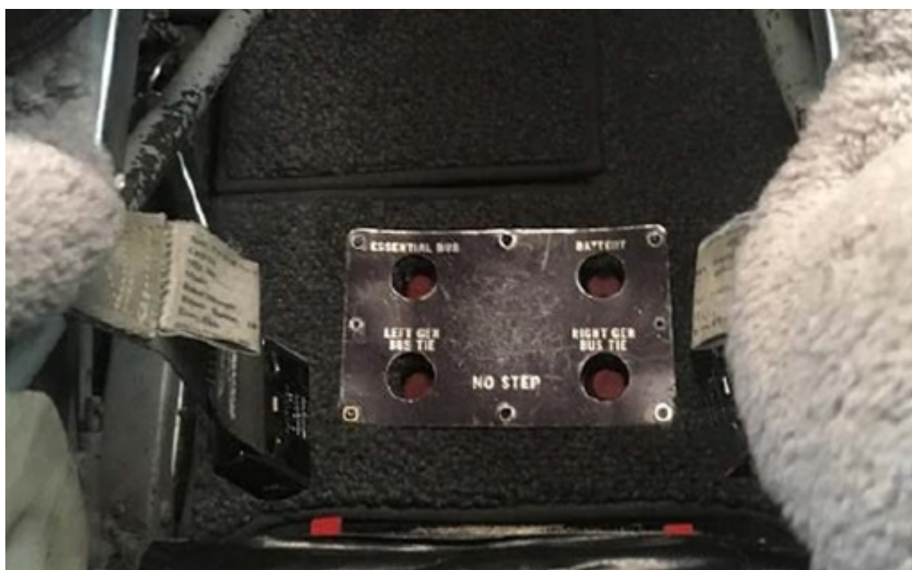
Figure 3 – Floor Mounted CB Panel – Interior (Typical of pre-1981 production)
