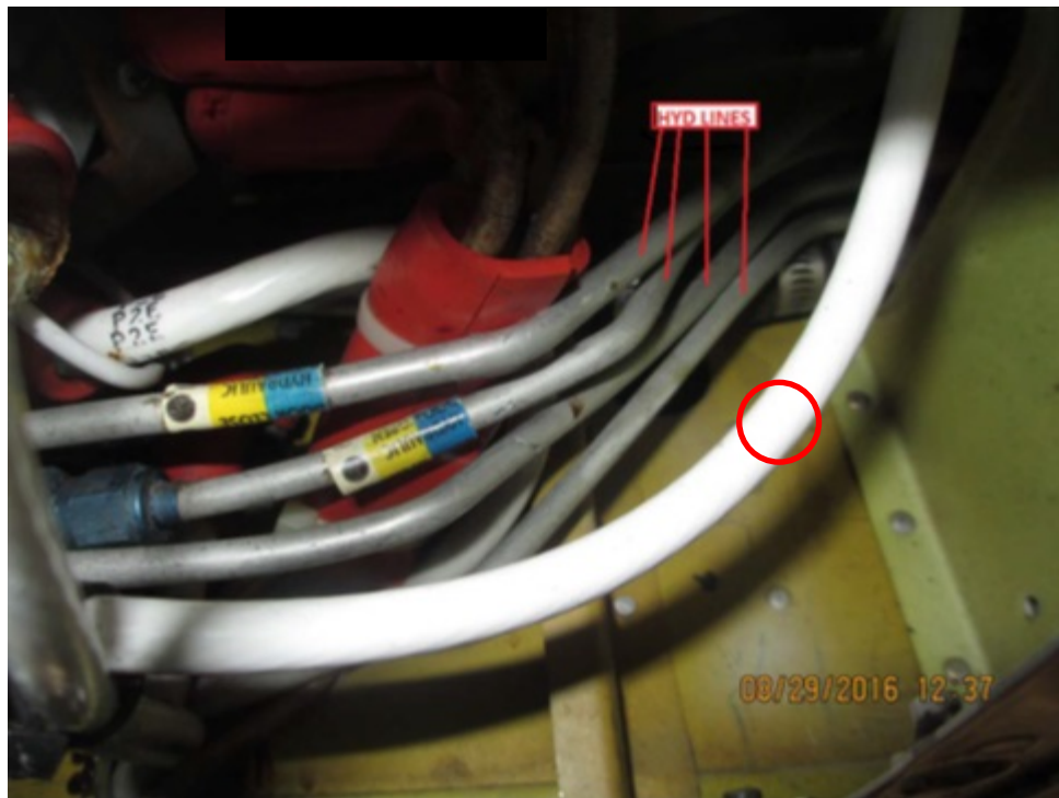
Figure 4 – View of the Hydraulic Lines in close proximity with electrical wires
